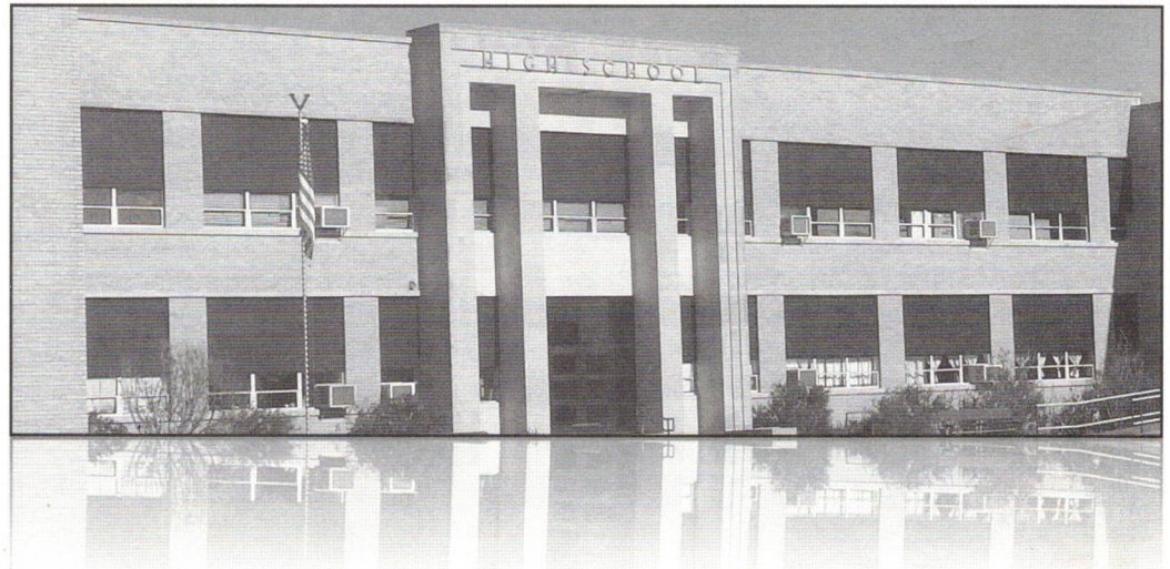
The Victoria Junior/Senior High School is shown with the new energy efficient material covering the top portion of the windows.
